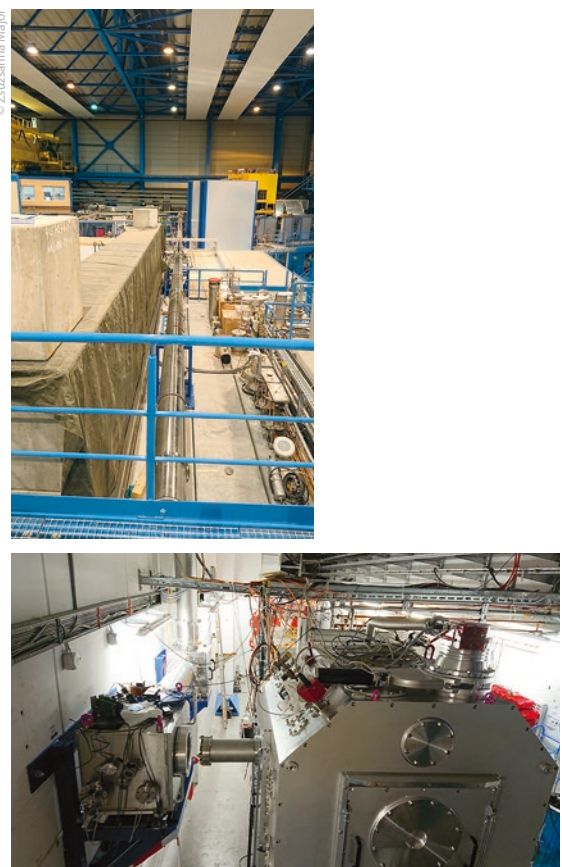
Figure 1: The newly commissioned PHELIX-HHT beamline. Top: the vacuum beamline for laser-beam transport traversing the experimental hall covering a distance of approx. 65 m between the PHELIX building and the HHT experimental area. Bottom: laser-beam transport and target chamber at HHT.
